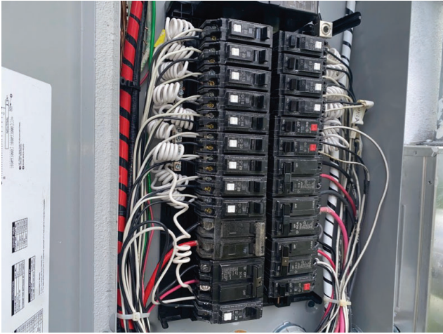
Exterior electrical circuit breaker box
