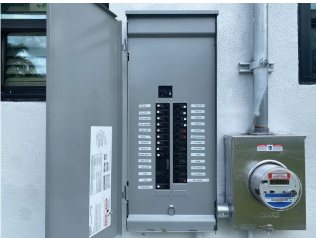
Exterior electrical circuit breaker box
