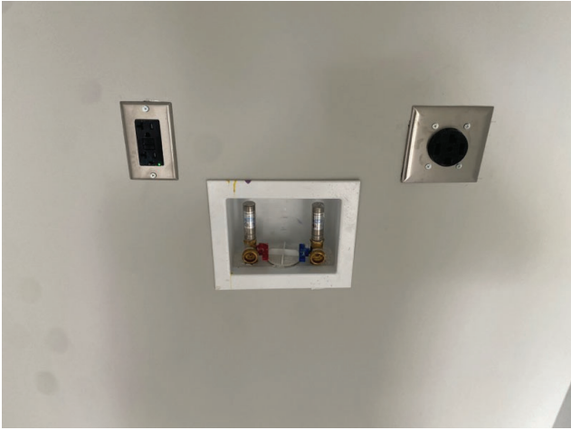
Washer plumbing hoses
