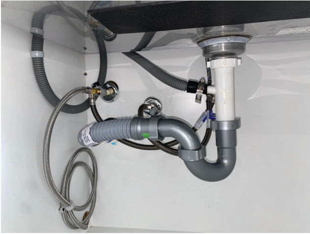
Kitchen plumbing component
