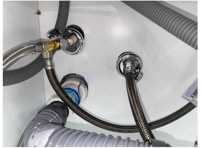
Kitchen plumbing component
