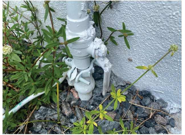
Main Water shut-off valve
