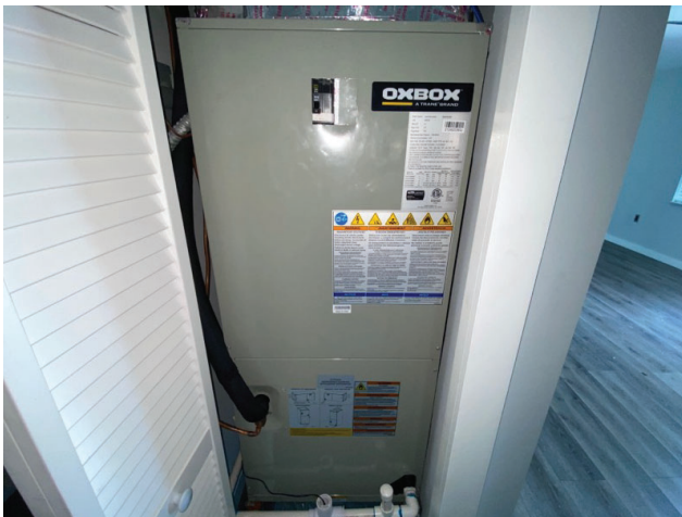
A/C Indoor air handler unit
