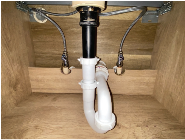
Bathroom plumbing component
