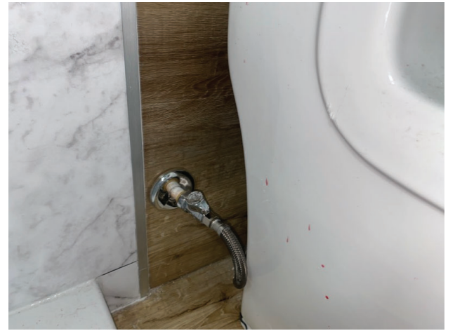
Bathroom plumbing component
