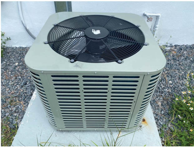
A/C Outdoor compressor unit
