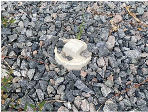
Pvc clean out for drainage
