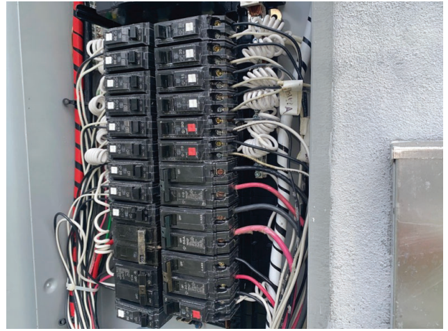
Exterior electrical circuit breaker box
