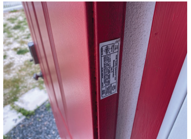
Rating label on front entry door
